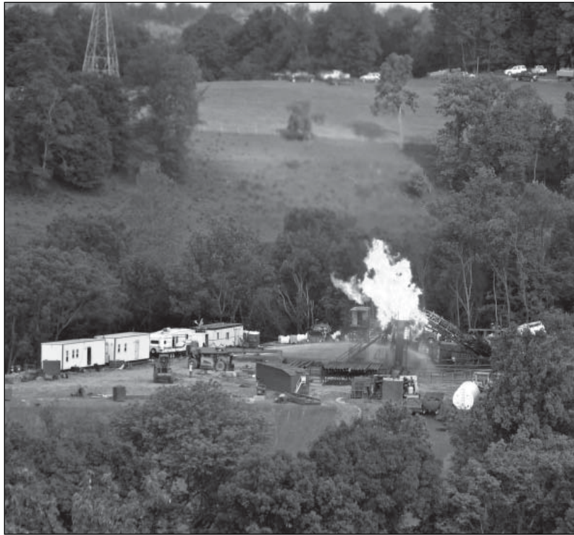
Figure 4.5. In June 2010, a drilling operation on a gas well in Marshall County, West Virginia, struck an abandoned coal mine triggering a blowout and explosion that injured seven workers (three seriously).
